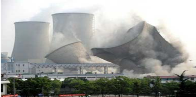
Two 90-m-high cooling towers collapse following a controlled explosion at the Huaneng Changxing Power Plant.
